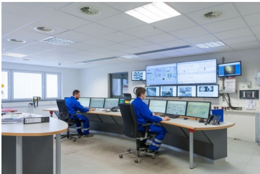
Picture 4: All information for operating and monitoring the entire process is collected in the central control room.
